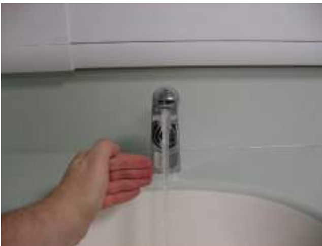
Figure 8.2 Sensor-operated tap fitted on a handwash basin; note there is no overflow.
